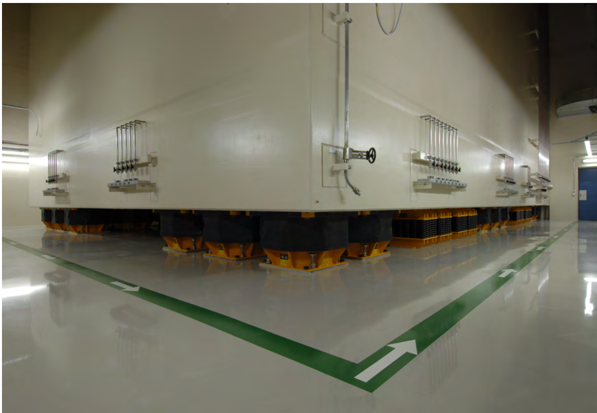
Figure 1-1: Outside view of the external spent fuel pool of the Gösgen nuclear power plant (KKG), equipped with seismic isolation.
