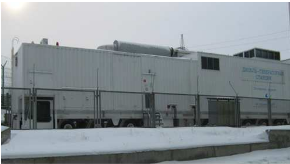
Fig. 2.3. Mobile emergency diesel-generator station, Novovoronezh NPP
