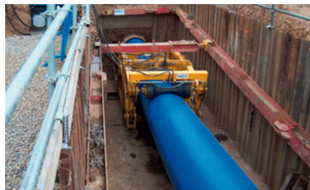
High density polyethylene liner being placed into host pipe (Photo: Swagnelining, UK).
