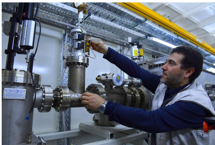
10 Messaoud Harfouche, XRF/XAFS beamline scientist, checking the reactor's XRF equipment. The XRF beamline hub uses the synchrotron light for research and training in a wide range of applications.
