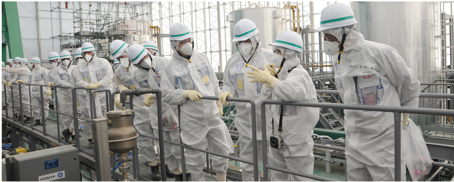
The IAEA decommissioning team listens to an explanation about the function of a purification system that removes almost all radioactive elements from contaminated water.
