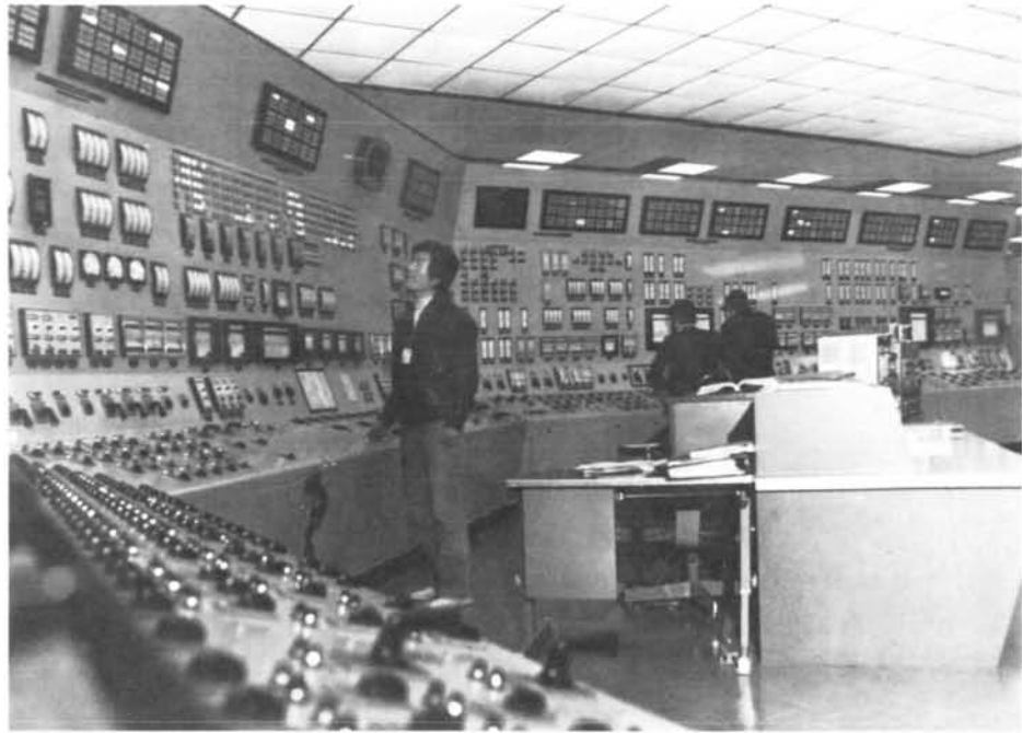
Computerized decision-aids for control-room operator support was one area drawing considerable interest at the international seminar on operational safety.
