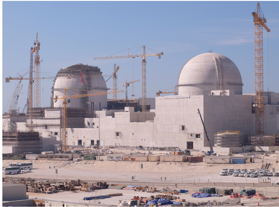
Barakah nuclear power plant, United Arab Emirates.
