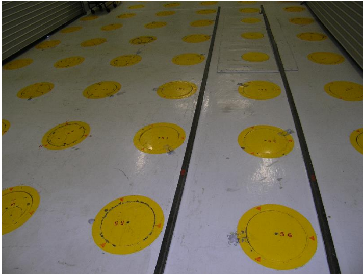
Figure D-3: Spent fuel storage facility. Kjeller site
