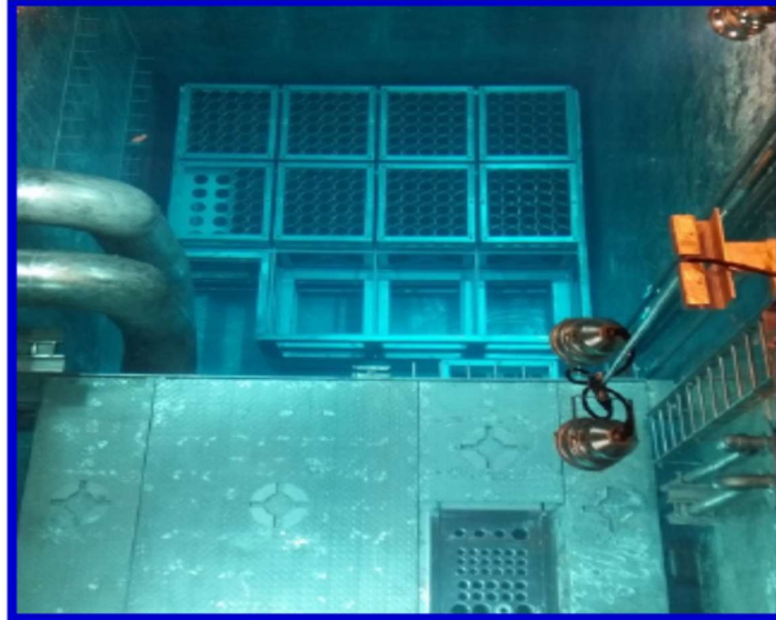
Figure B.1 Overview of the SNF Storage Racks
