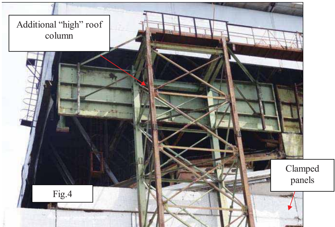
Figure 4 Turbine Building view from outside of wall panel failure in “high” roof zone next to gridline 50
