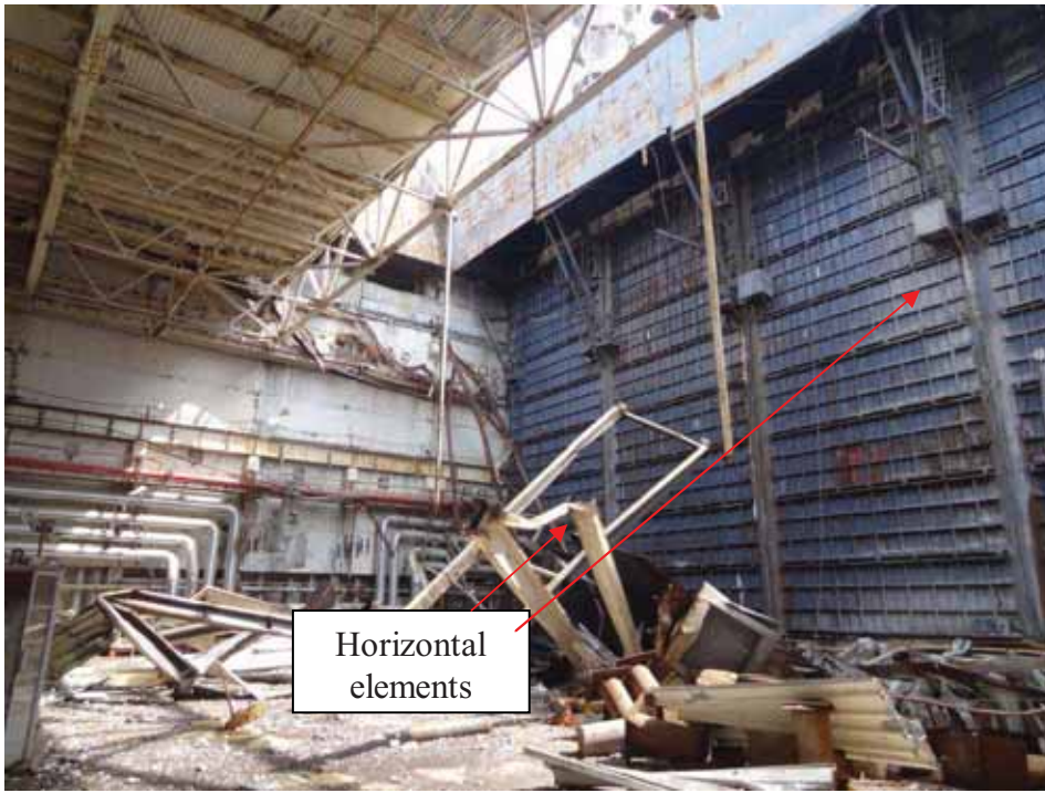
Figure 3 Turbine Building view of area of collapsed roof section
