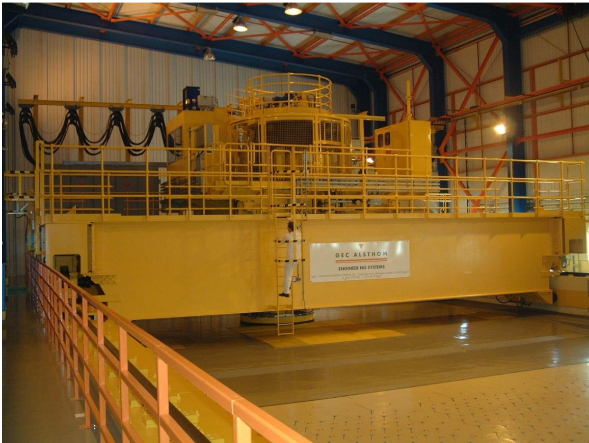
Figure G.1-2 Re-fuelling machine in the Spent Fuel Interim Storage Facility
