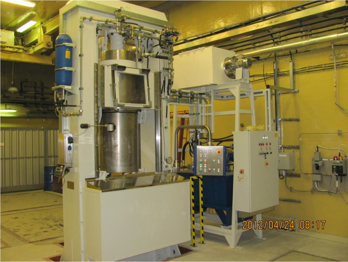
Figure D.2.4 – 2. Waste compressor machine
