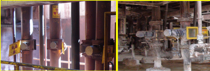
Fig. 1 - Nuclear gauges in radioactive facility.
