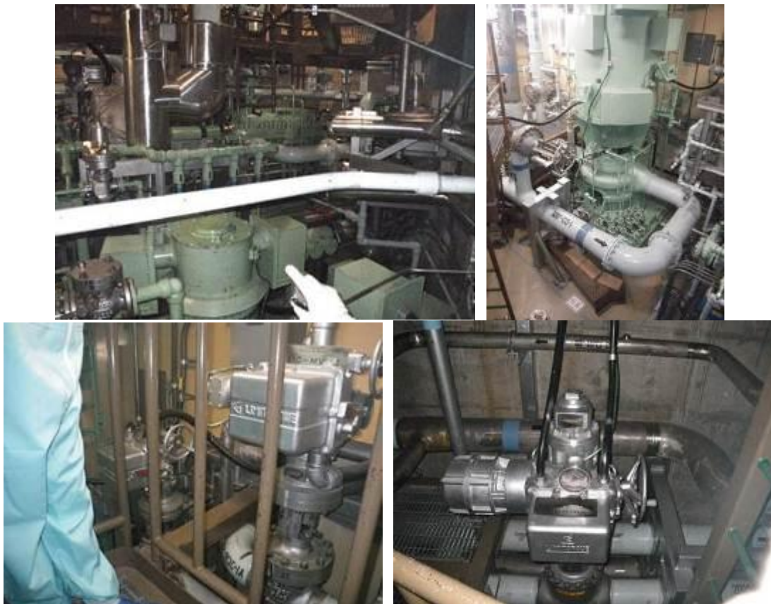
Figure 7-2 RCIC Steam Driven Pump (upper left), Low Pressure Core Spray Pump (A) (upper right), and Motor Operated Valves for these systems (lower)
