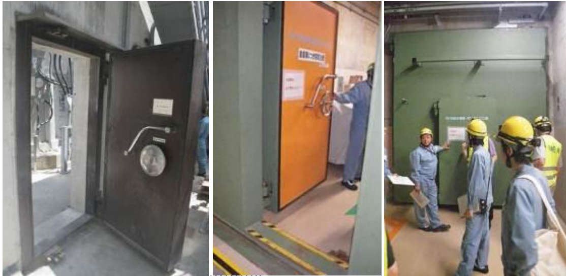
Figure 7-36 Water Tight Door in Seawater Pump Pit (left) and in RCW HX Room (middle and right) at Unit 2
