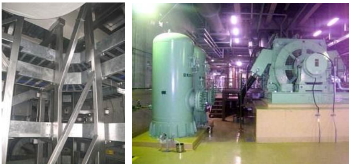
Figure 7-5 Sample of Cable Tray Supports (left) and Emergency Diesel Generator (right)
