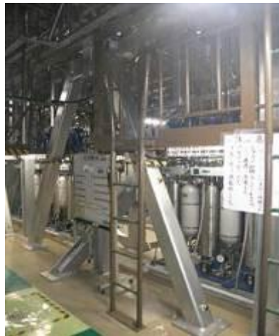
Figure 7-1 Hydraulic Control Units
