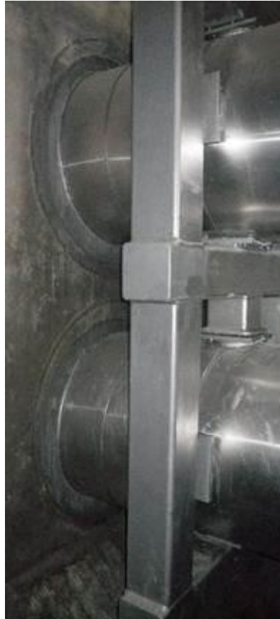
Figure 7-35 Pipe penetration from the RSW pit to the RSW trench The resin sealant (dark gray rings between wall penetrations and RSW pipes) is installed after March 11 Tsunami at Unit 2.
