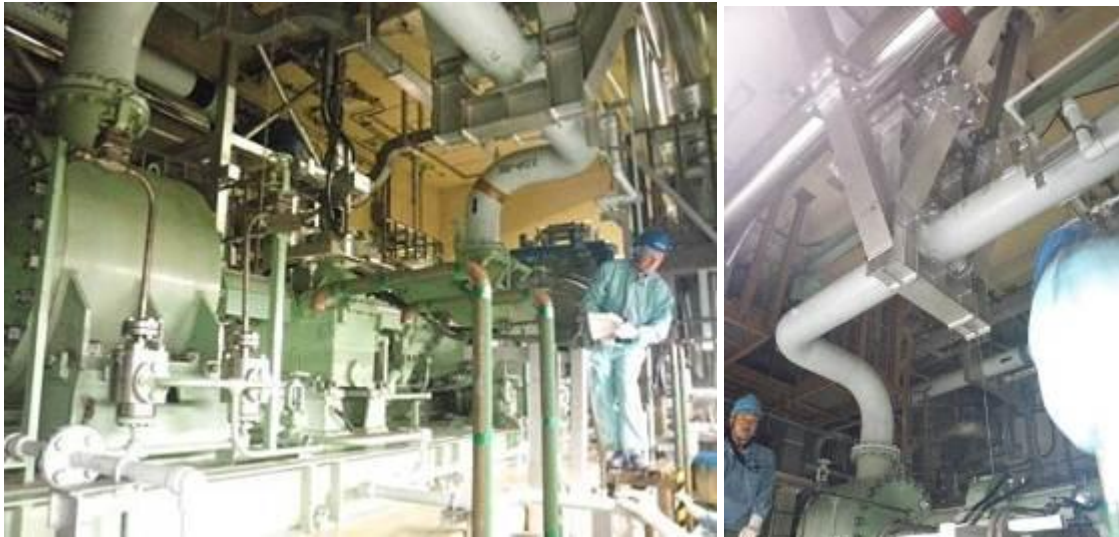
Figure 7-3 High Pressure Core Injection Pumps (left) and its pipe support (right) in Unit 1
