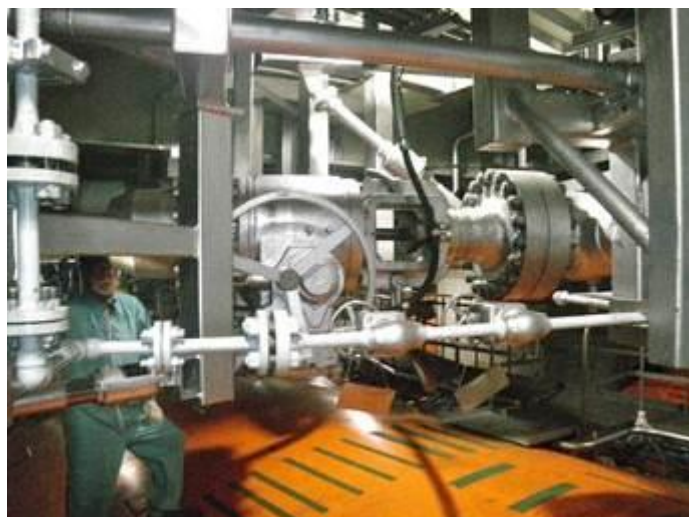
Figure 7-7 In Containment Above Torus – showing seismic supports
