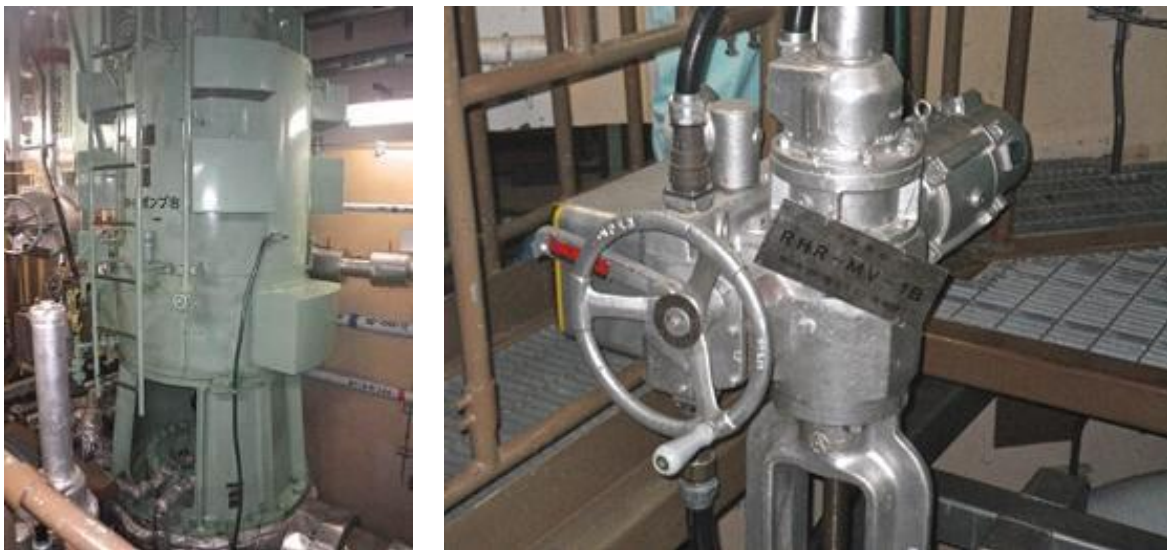
Figure 7-6 RHR Pump and RHR Motor Operated Valve
