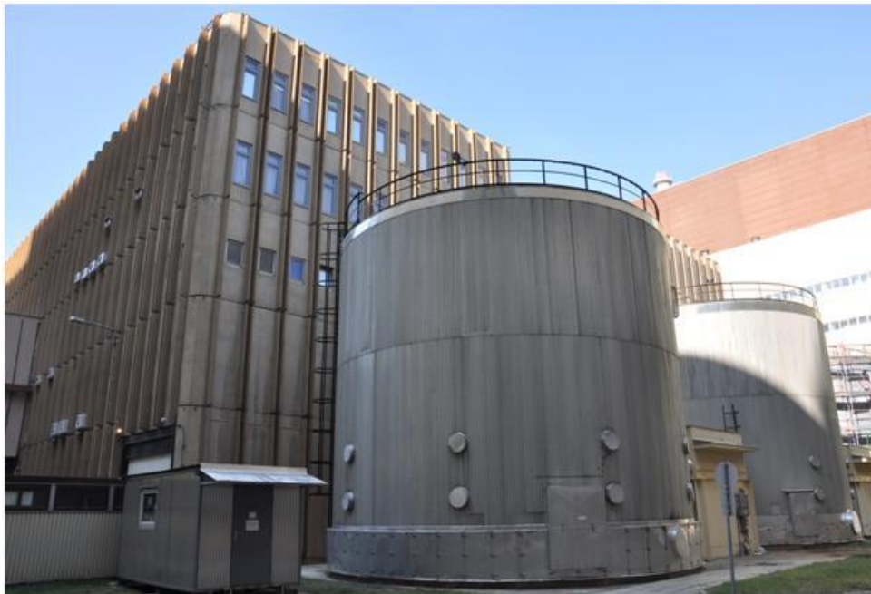
Figure 2-3: Demineralised water tanks of Installation II
