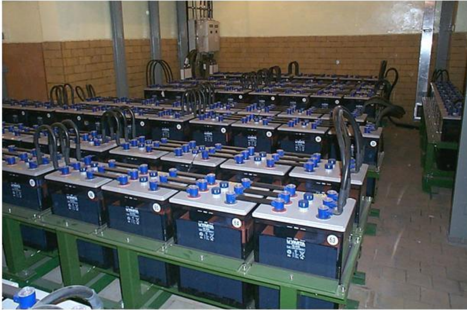
Figure 2-1: Batteries of direct current supply of a unit
