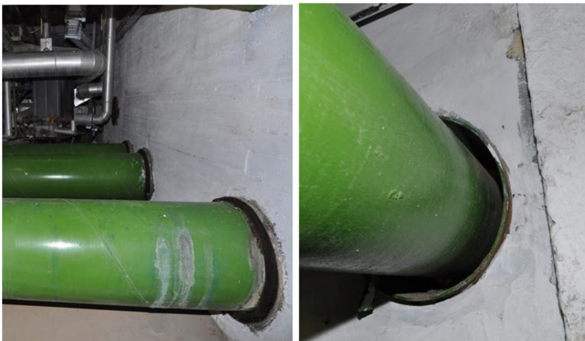
Figure 2-6: Underground connection point of the essential cooling water system to the main service building
