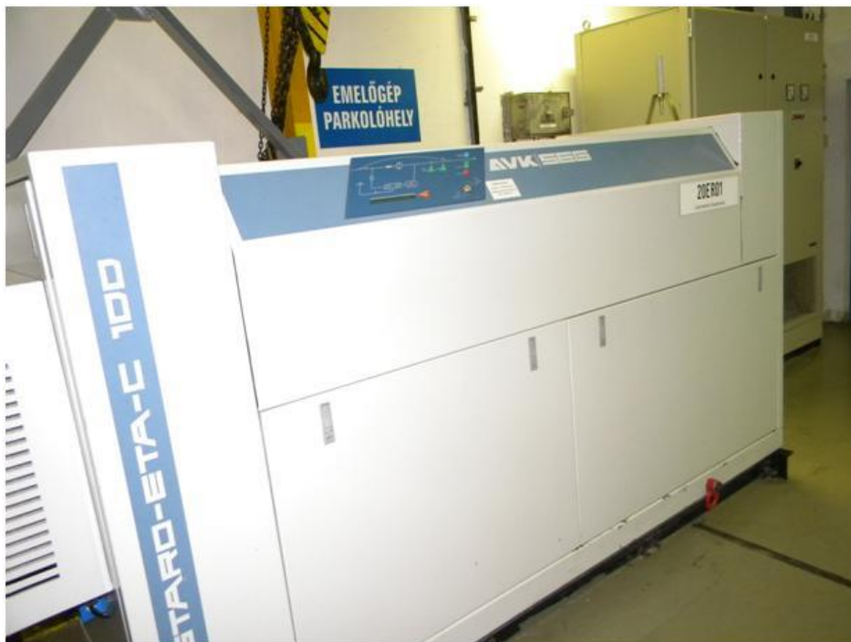
Figure 2-2: Inverters of direct current supply of a unit
