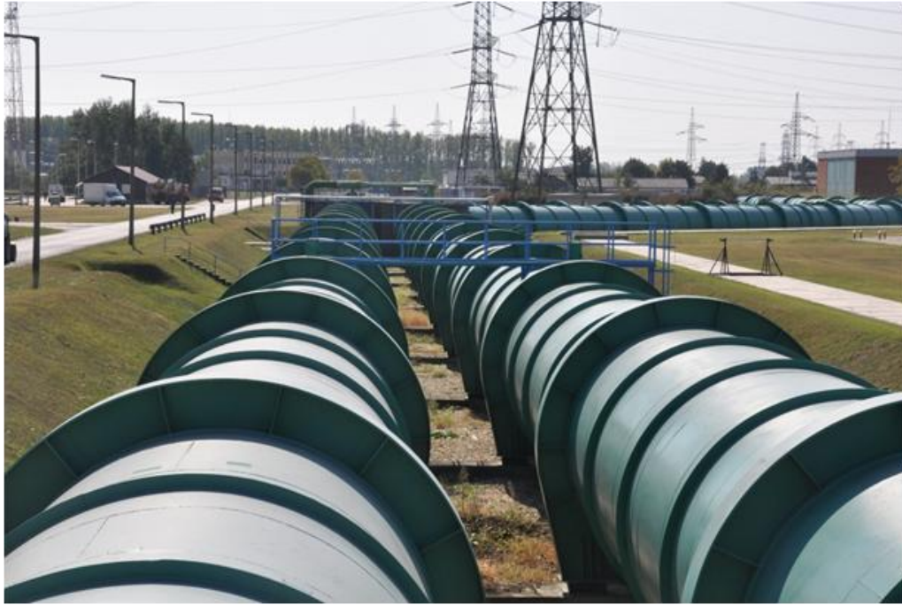
Figure 2-7: Courtyard pipelines of the main condenser cooling water system
