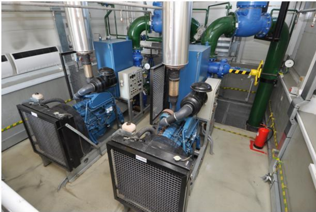
Figure 2-8: Diesel-driven fire water pump station
