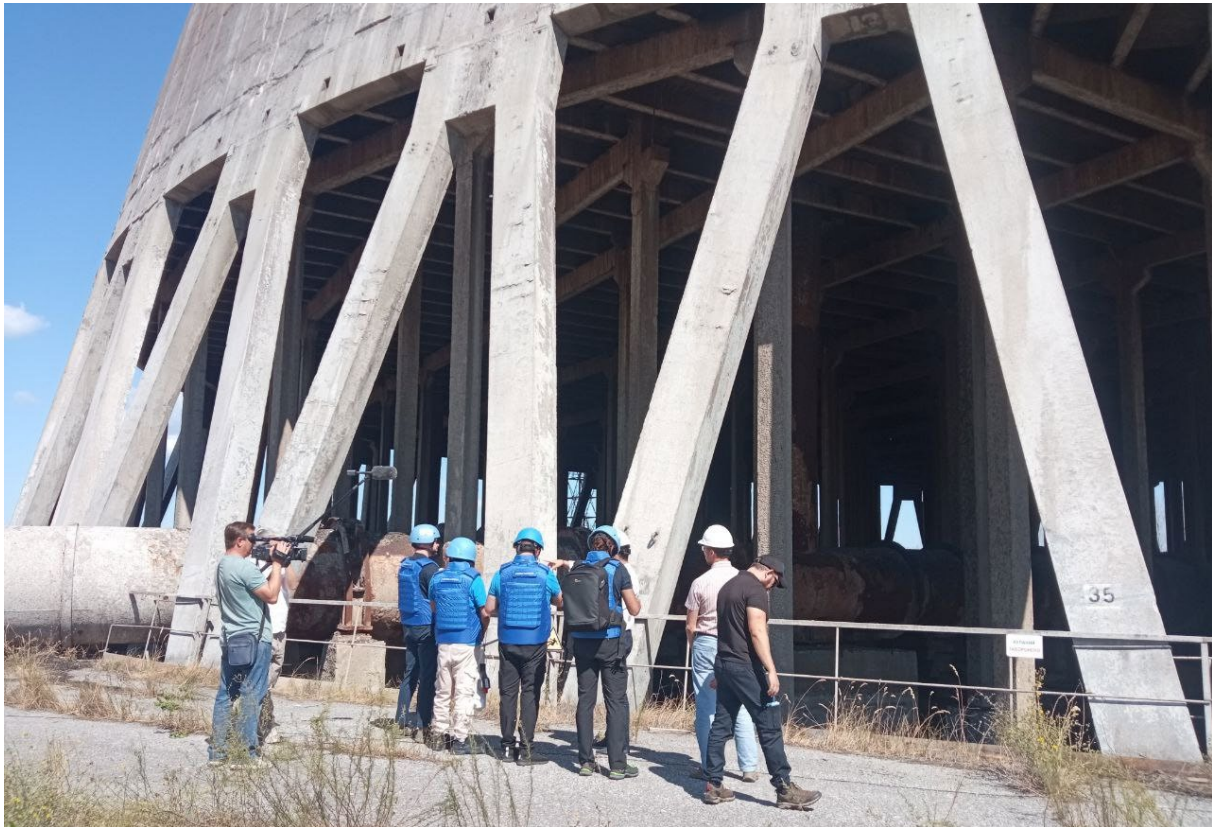
ISAMZ observing the damage at the cooling tower on 12 August 2024. (Photo: ZNPP)
