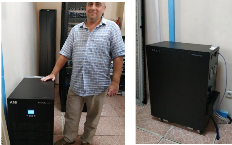
Uninterruptible power supply unit delivered to the Ukrainian Hydrometeorological Centre of the State Emergency Service of Ukraine on 8 July 2024, procured using extrabudgetary funding from Switzerland. (Photo: Ukrainian Hydrometeorological Centre of the State Emergency Service of Ukraine)
