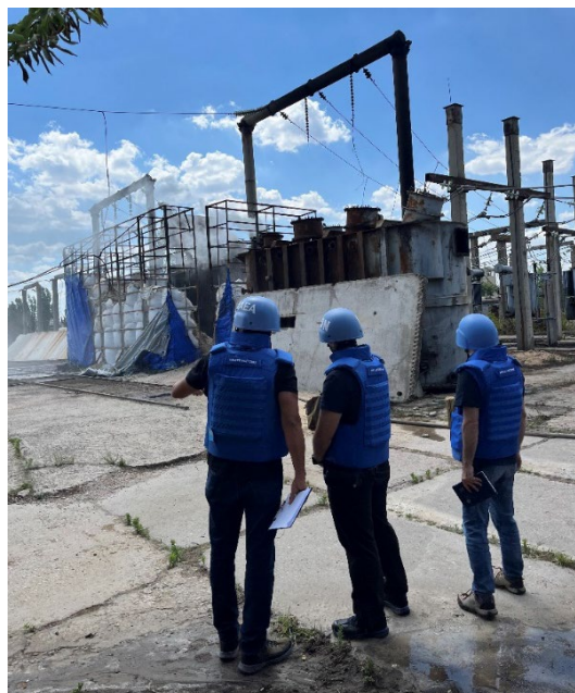
ISAMZ observes the damage at the Raduga electrical substation on 20 June 2024.
