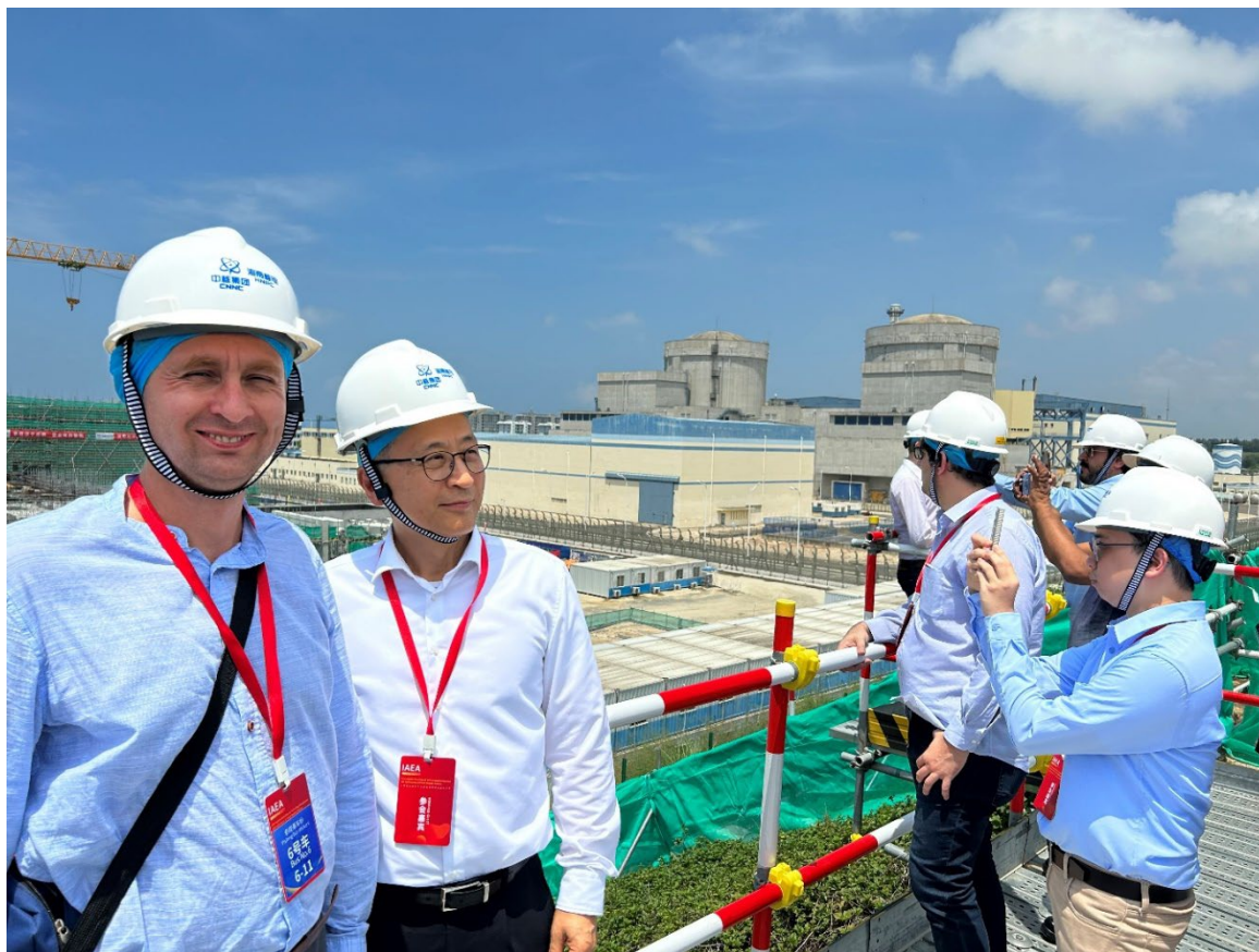
Fig. B.2. A visit to a NPP construction site held on the margins of the combined Interregional Workshops on Technology Development and Applications and the Generic User Requirements and Criteria for SMRs, held in China in September 2023. (Source: IAEA)
