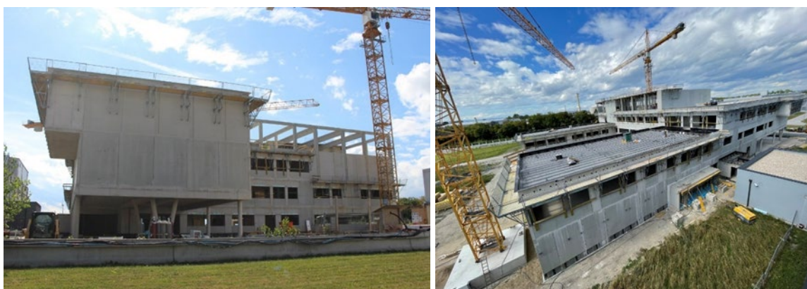
FIG. B.1. Works on the FML2 façade and roof insulation, September 2023. (Source: IAEA)
