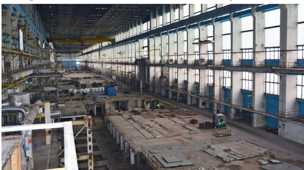
Dismantling activities in the turbine hall of the Kozloduy NPP Units 1-4 is nearing completion, Kozloduy, Bulgaria, November 2019. (Photo: State Enterprise Radioactive Waste, Bulgaria)
