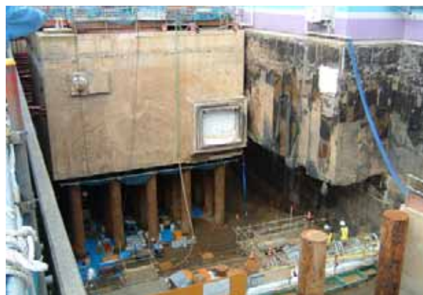
FIG. 2. Removal, cleaning and replacement of oil contaminated soil below the pile foundation of a non-safety related structure at the Kashiwazaki-Kariwa nuclear power plant.
