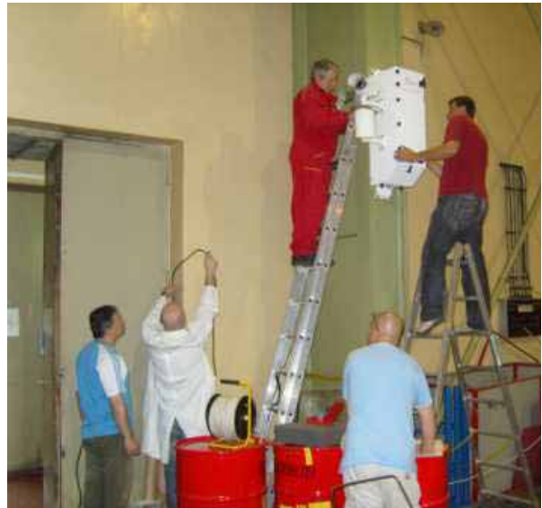
FIG. 2. Installation of remote monitoring equipment to improve the physical protection of a nuclear facility.
