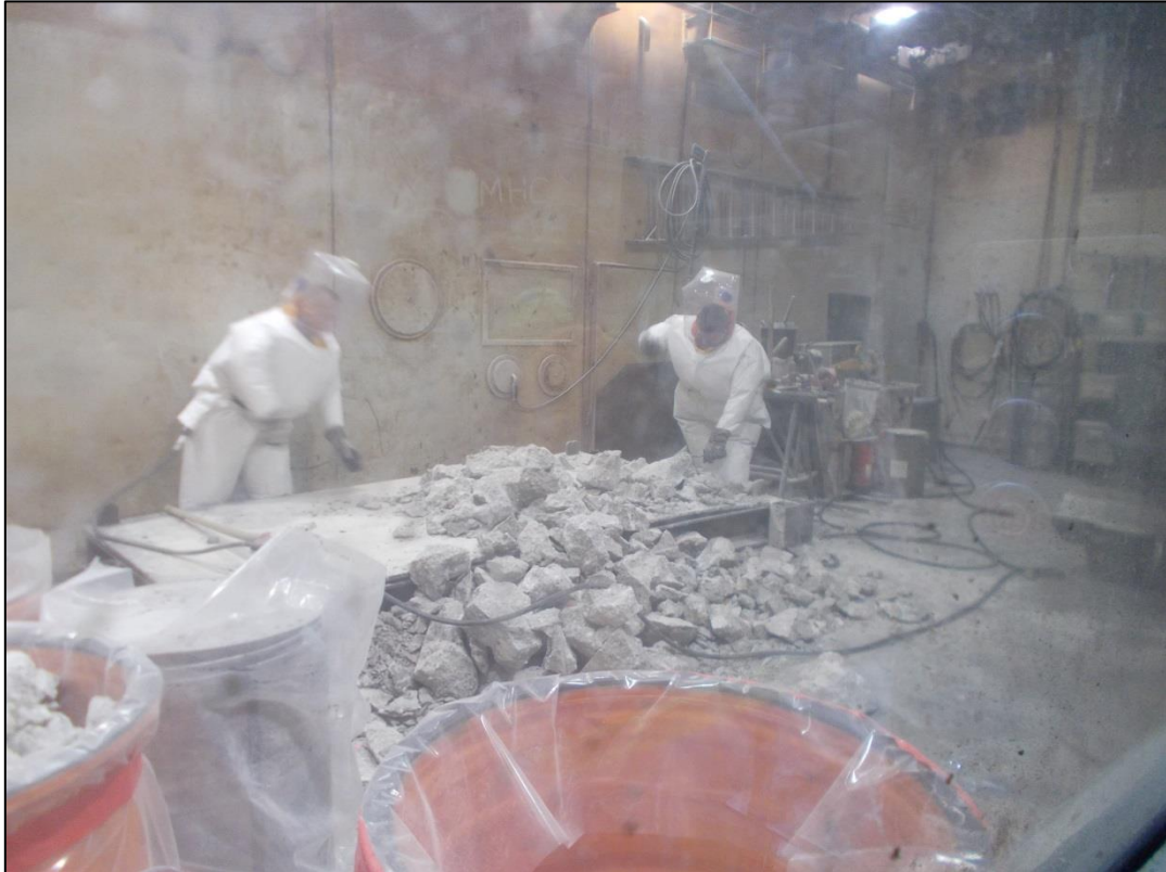
Waste treatment facility at KTE site ( courtesy of KTE )
