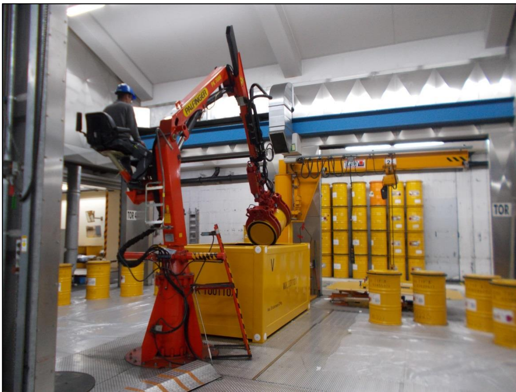
Loading of drums of radioactive waste into an ISO container at the KTE storage facility (courtesy of KTE)
