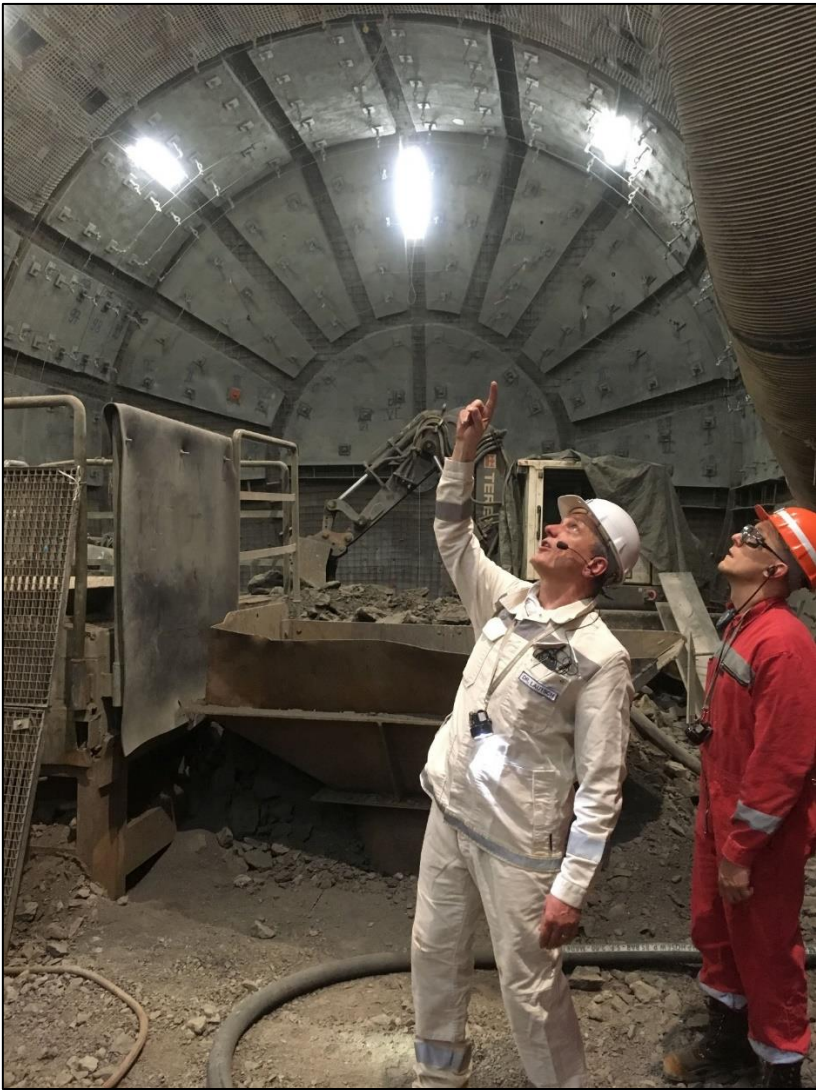
A view of disposal facility excavations at Konrad illustrating the large diameter of the tunnels, and showing the use of extensive rock support in the form of rock bolts and iron mesh (courtesy of BGE).
