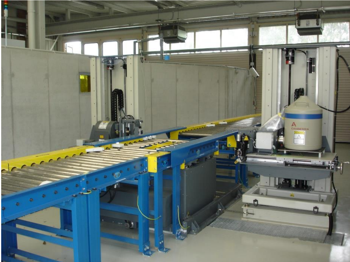
Figure 9 Waste Assay System in the measuring facility at Seibersdorf, © NES
