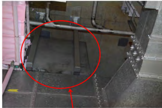
Unit 5 southwest overflow chamber
