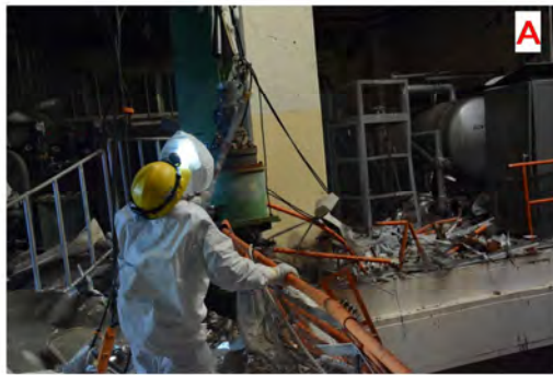
Witness standing position during Water leak
