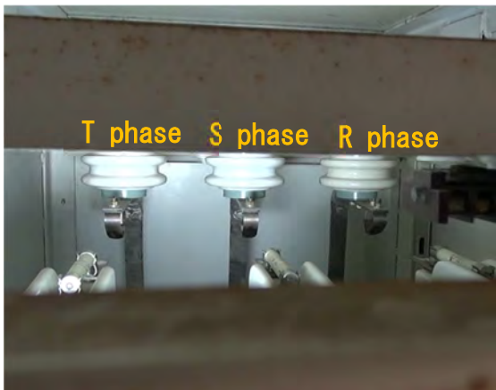
Insulating resistance measuring points on top of Cabinet 5
