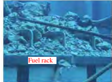
Photo③ Deposits on the fuel storage racks
