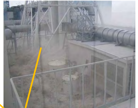
Main stack of the turbine building's ventilation system
