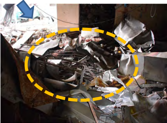
Photographed by the NRA on July 12, 2013 Floor damage in the northwest area of the 3rd floor
