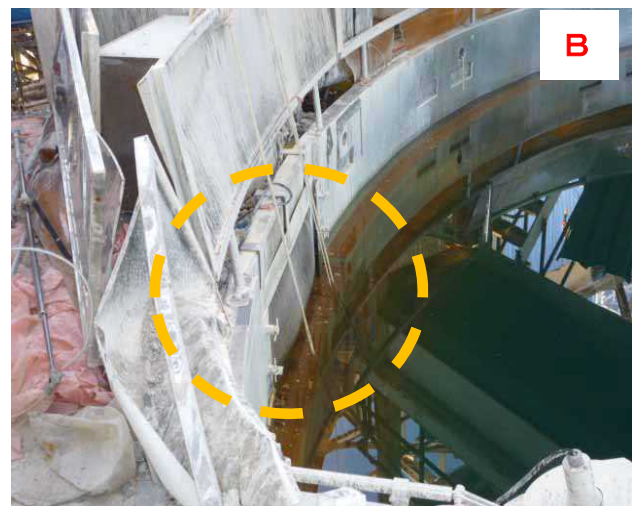
Deformation of the exhaust port net of the exhaust duct above the reactor well on the 5th floor (deformed outward) (photographed by TEPCO on November 8, 2011)
