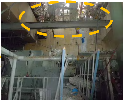
Photographed by TEPCO on November 8, 2011 Ceiling damage in the southwest area of the 4th floor
