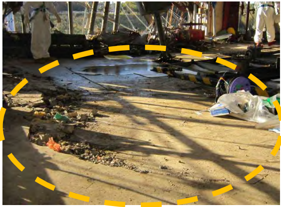
Photographed by TEPCO on November 8, 2011 Floor damage in the southwest area of the 4th floor
