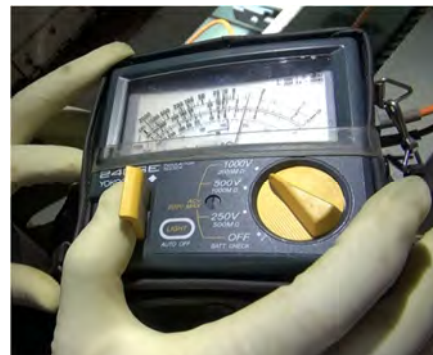
2.7 MΩ between T and R phases
