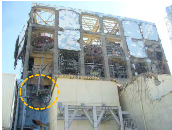
Photographed by TEPCO on March 18, 2011 Complete destruction of the wall west of the staircase in the northwest area of the 3rd floor
