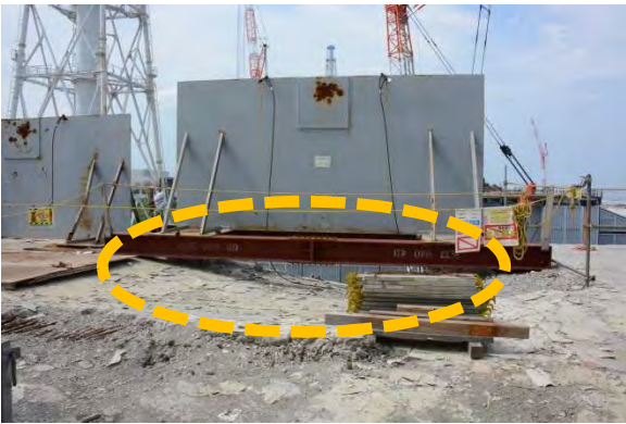
Photographed by the NRA on July 11, 2013 Downward deformation in the north area of the 5th floor
