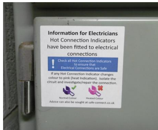
Figure 3.1: Cable hot connection indicators
