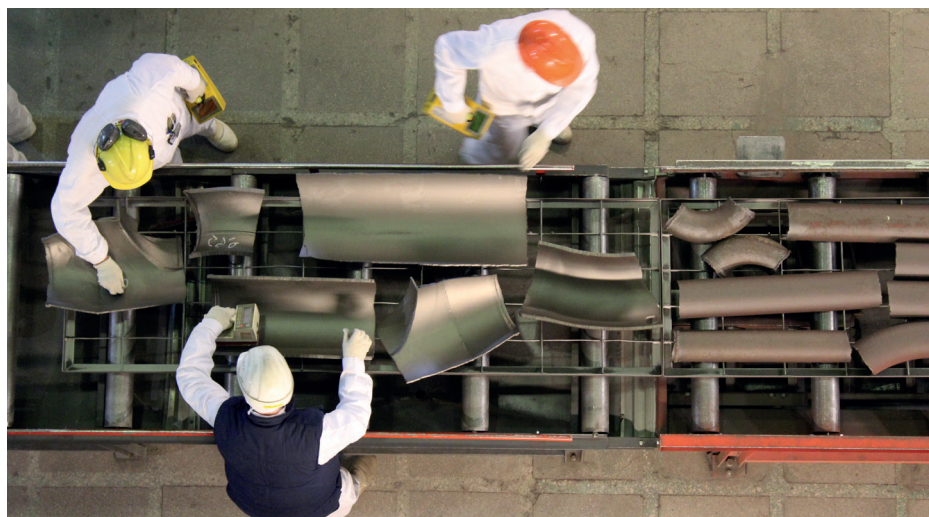
Workers dismantling a turbine hall measure scrap metal for traces of radiation.
