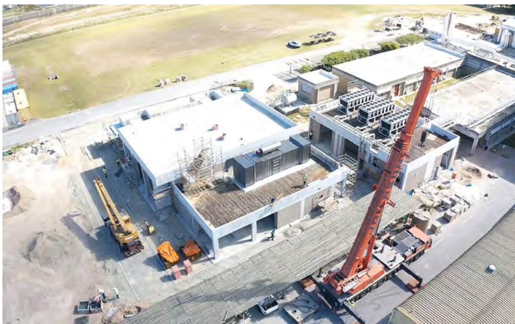
FIG. 9: Bird's eye view of the new mechanical and electrical plant rooms under construction
