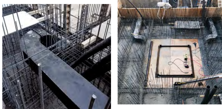
FIG. 13. Ins and outs ventilation ducts from the vault
