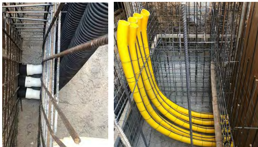
FIG. 14. General services piping
