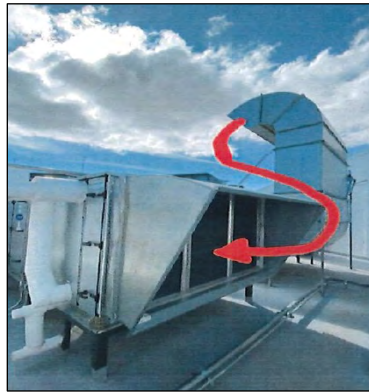
FIG. 1. Initial inlet and outlet pipe HVAC system arrangement installed in the building and possible radioactive gas trajectory entering production main floor.
