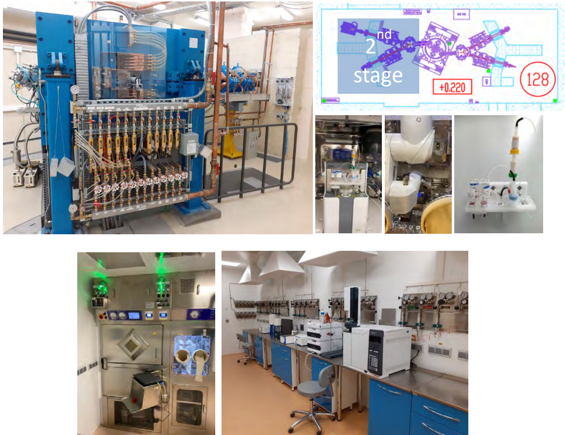
FIG. 9. Cyclotron and radiopharmaceutical production facility with analytical equipment
