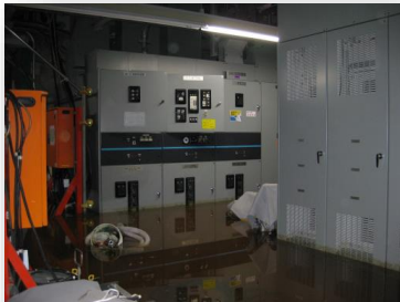
Power Center (P/C)
