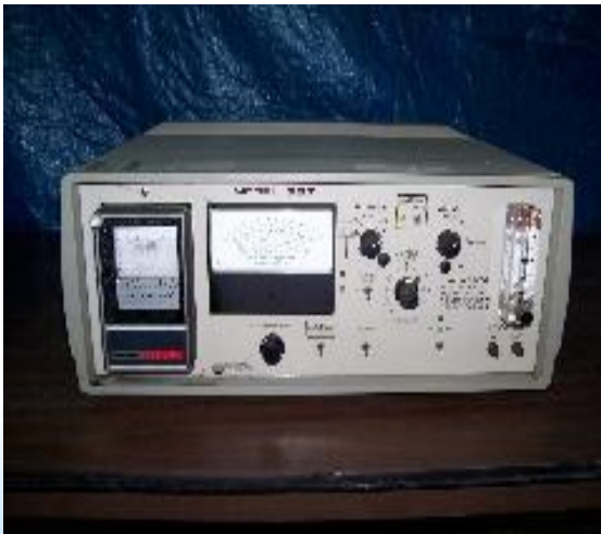
Installed H-3 monitor
