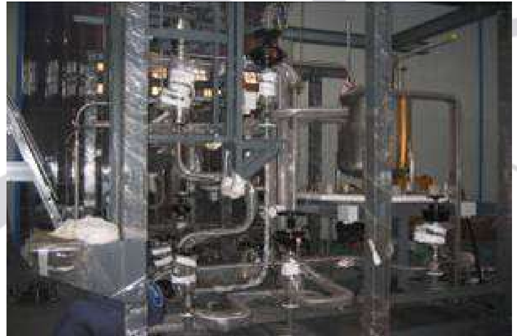
Sodium Treatment Facility at Creys Malville (courtesy of EDF, France).
