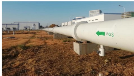
A pipeline carrying heated water from the Haiyang plant (Image: SPC)
