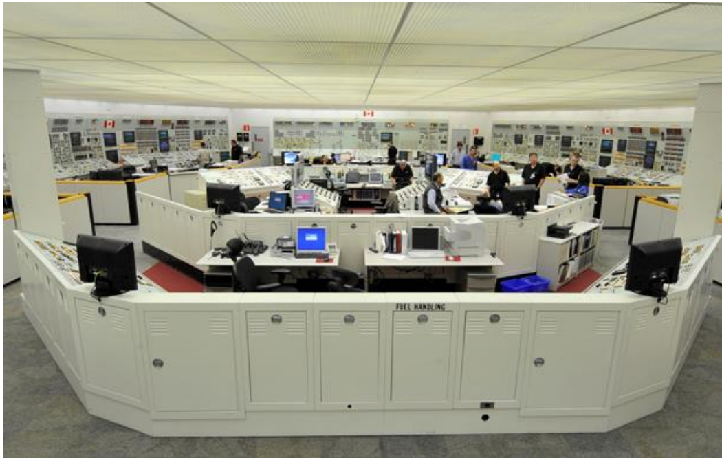
Figure 4A: Main Control Room Bruce Nuclear Generating Station B, Canada: source Brucepower.com
