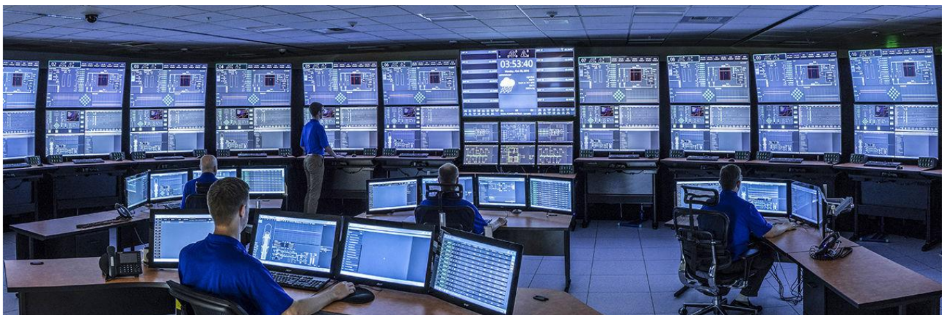
Figure 4B: Main Control Room NuScale Power, USA: source NuScalePower.com
