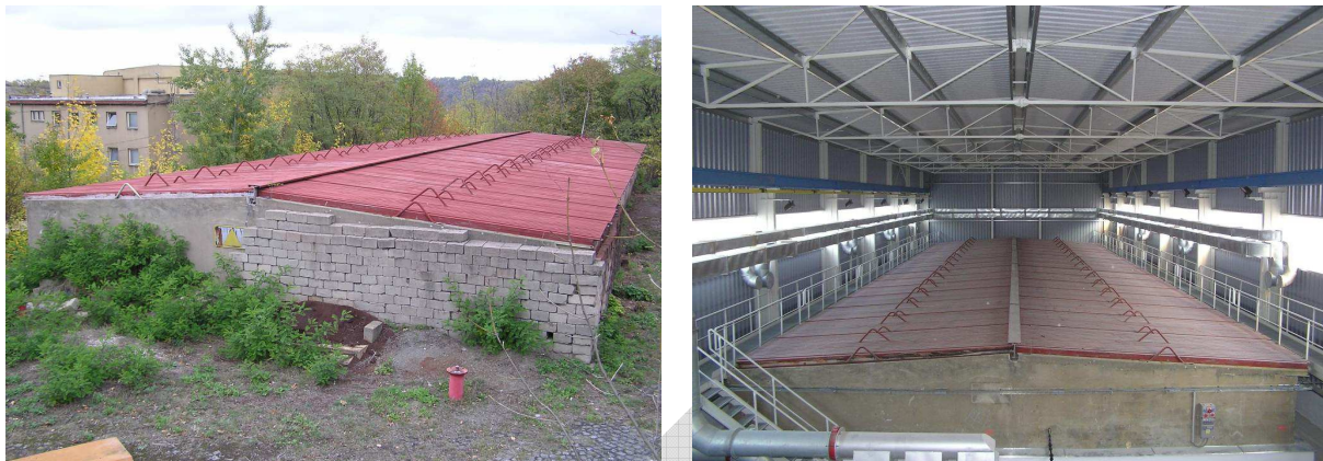
FIG. III-2. Original condition of the storage facility (left), and following the installation of an overbuilding and other systems (right)
