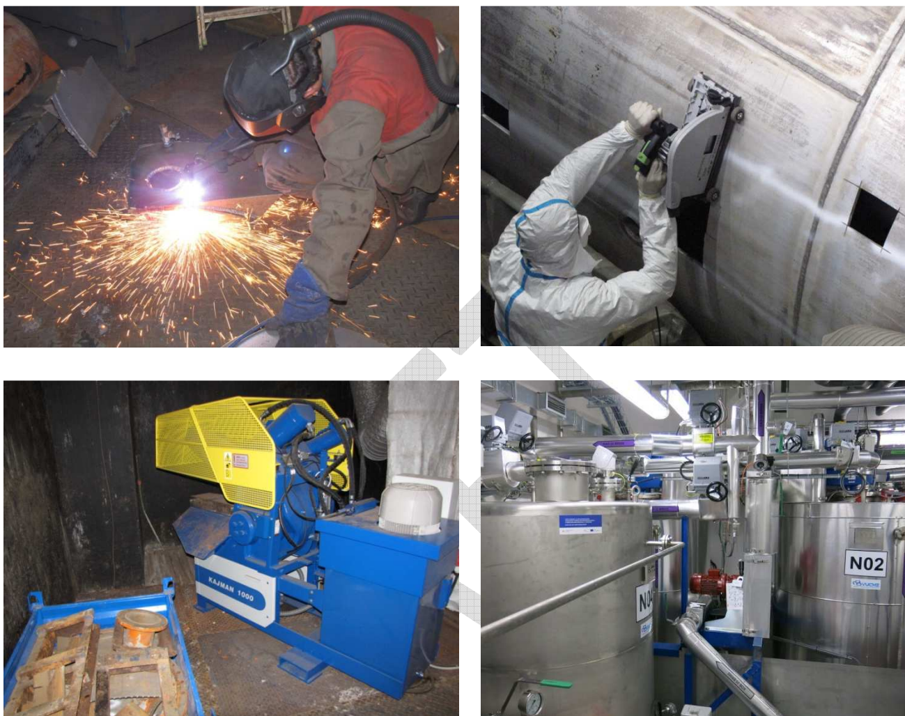
FIG. III-4. Examples of techniques planned for use in decommissioning operations, i.e., plasma cutting, circular saw cutting, hydraulic power shears for segmentation, evaporation system for secondary liquid waste processing
