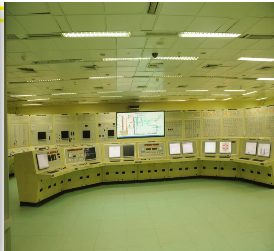
Main Control Room
