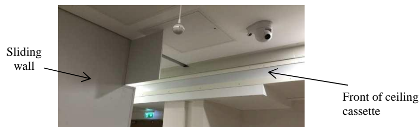
FIG.3. Ceiling cassette assembly which penetrates the concrete wall.
