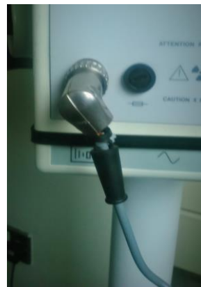
FIG. 5. Damaged strain release collar
