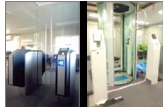
Access Control System
