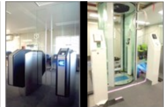
Access Control System
