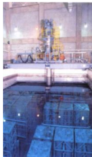
Spent Fuel Pond
