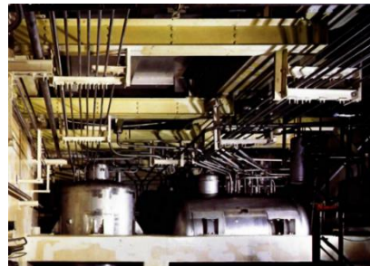
U Nitration Tanks
