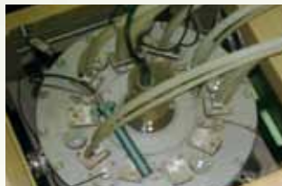
Reactor vessel head
