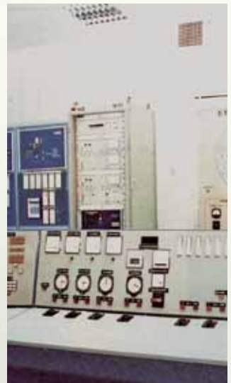
Reactor control panel
