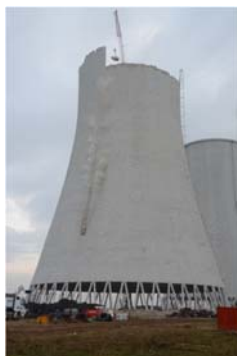
FIG. A-6. Demolition of V1 Bohunice NPP cooling towers, Slovakia, October 2017. (Photo: JAVYS).
