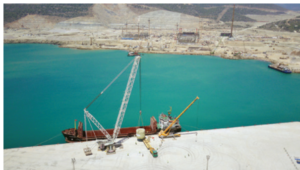
Construction site of the Akkuyu nuclear power plant, Turkey, August 2020. (Photo: Akkuyu Nuclear JSC)
