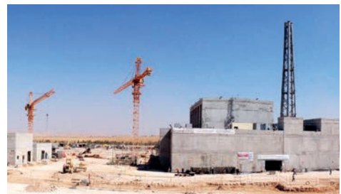
Close to complete construction of the Jordan Research and Training Reactor (JRTR), with the 1st criticality achieved in April 2016. Source: JAEC.
