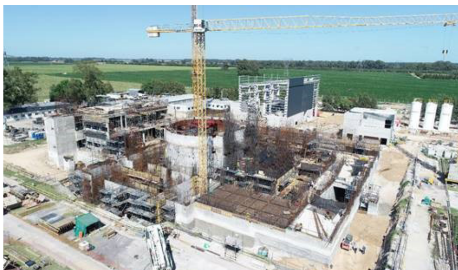
FIG. A-2. CAREM is at an advanced stage of construction at a site adjacent to the Atucha II/Néstor Carlos Kirchner NPP in Argentina, for operation by 2024 with a view to producing 30 MW(e) as a prototype demonstration. (Photo: CNEA)
