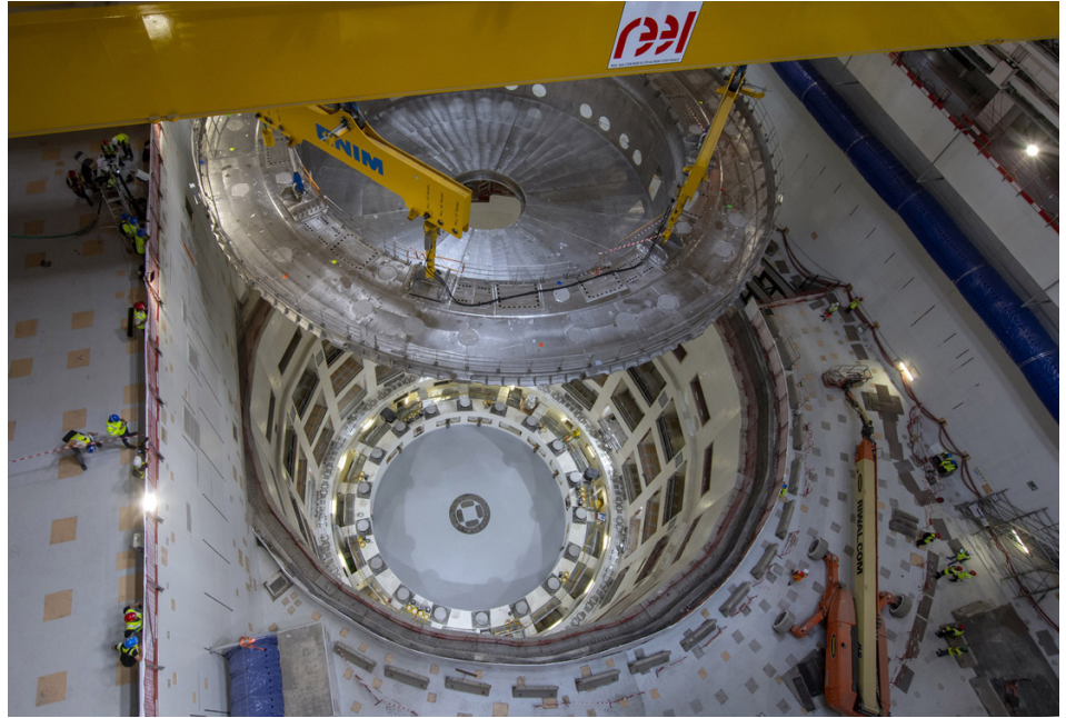
FIG. A-5. The 1250-tonne cryostat base was the first large-scale component to be installed at the bottom of the 30-metre-deep Tokamak assembly pit. (Photo: ITER Organization)
