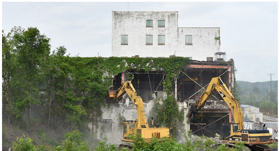
FIG. C-3. Progress in remediation work made at the site formerly known as the Oak Ridge Gaseous Diffusion Plant in Oak Ridge, Tennessee, United States of America. (Photo: DOE)
