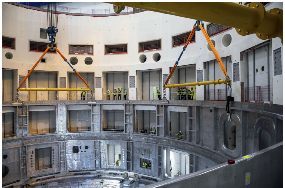
FIG. A-6. After the cryostat base was installed, the 375-tonne cryostat lower cylinder was lowered to the bottom and welded to the base. (Photo: ITER Organization)
