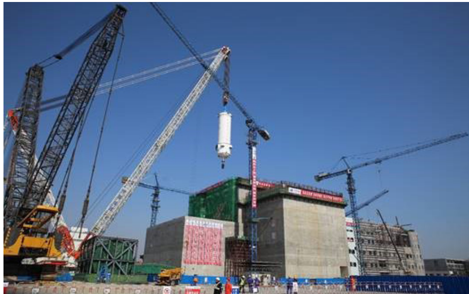
FIG. A-1. The HTR-PM in China undertaking system hot functional commissioning, with a view to starting commercial operation in 2022. (Photo: Institute of Nuclear and New Energy Technology, Tsinghua University, China)
