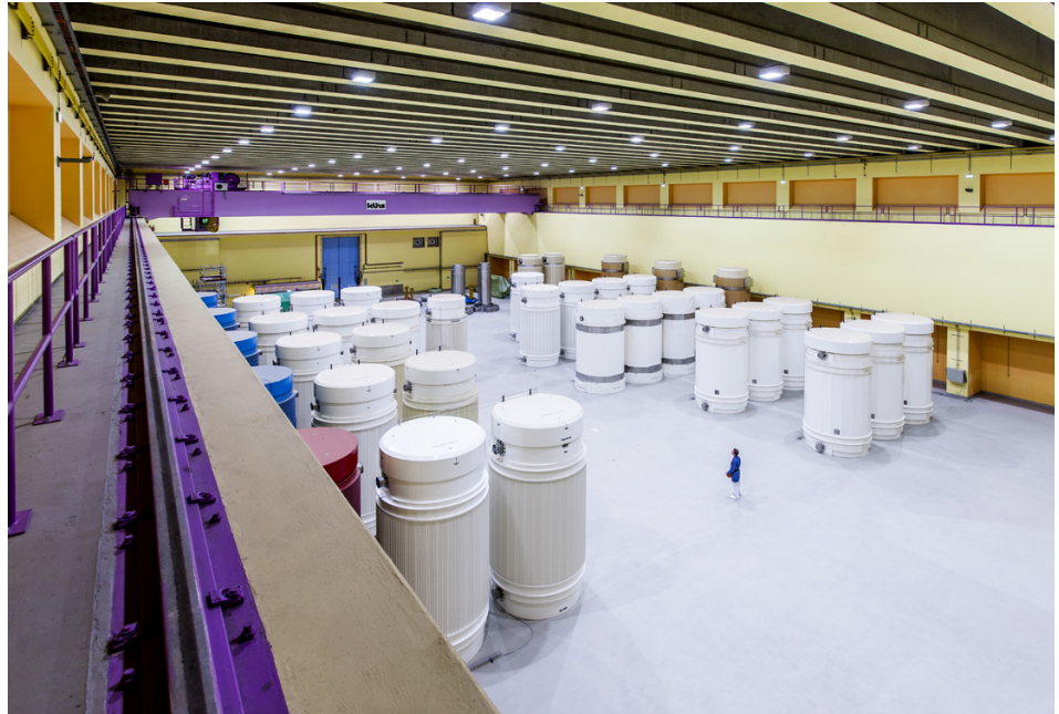
FIG. C-5. The cask storage hall at ZWILAG in Switzerland is used to store vitrified high level waste from reprocessing plants and spent fuel elements from Swiss NPPs. (Photo: ZWILAG)
